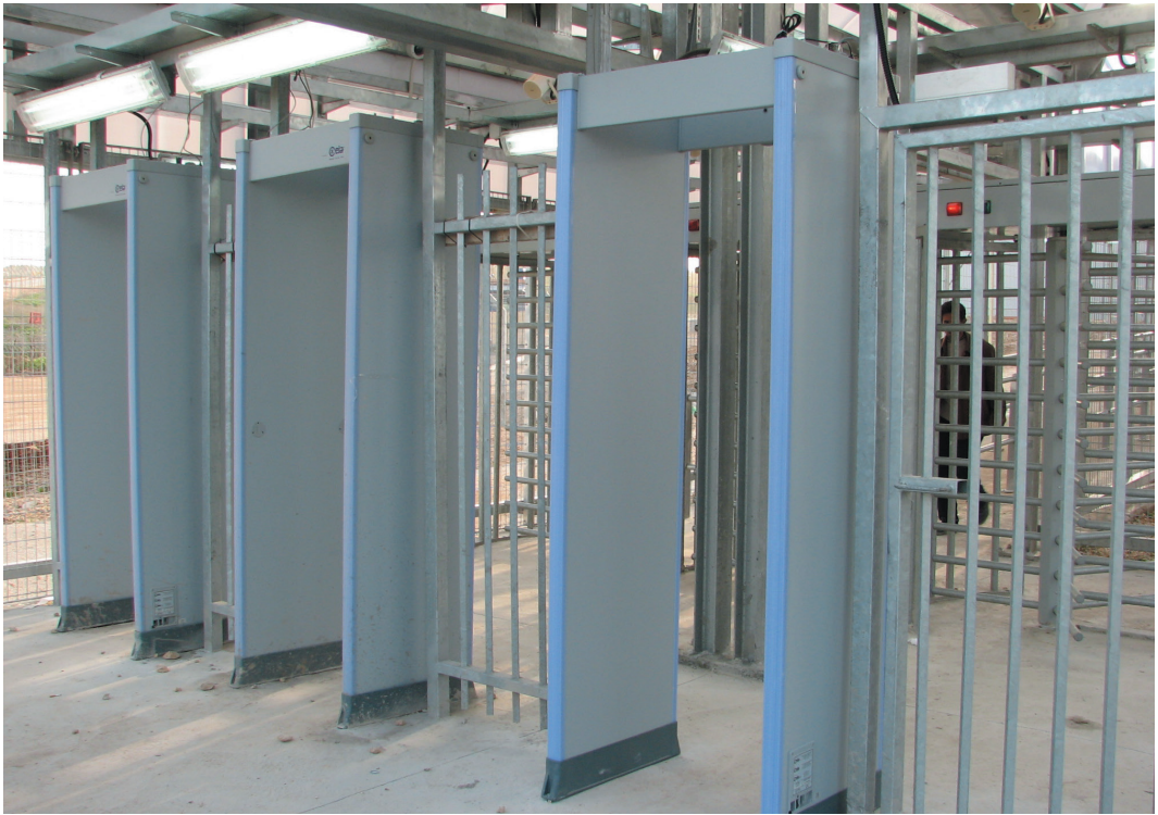
The third phase of pre-screening before entering the terminal building at Einab
